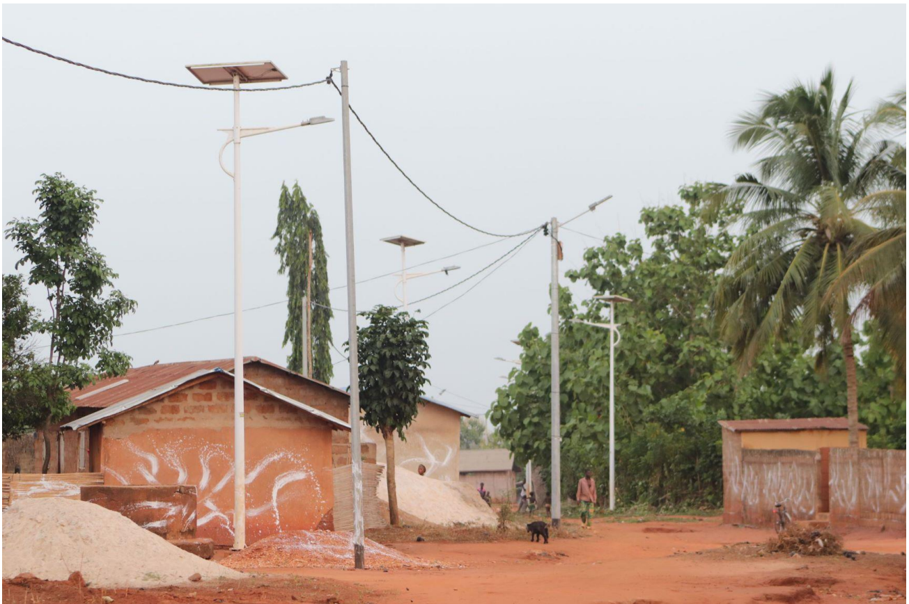
Photo: Solar street lighting at the BBOXX and EDF “Tomorrow’s Connected Community” in Togo
